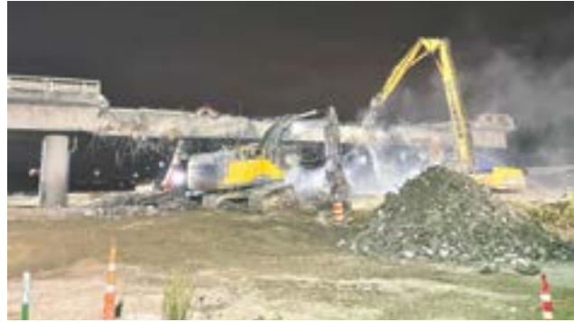
In late September and into October, WSDOT closed I-5 overnight to demolish the old, out-of-use 70th Avenue East bridge.
