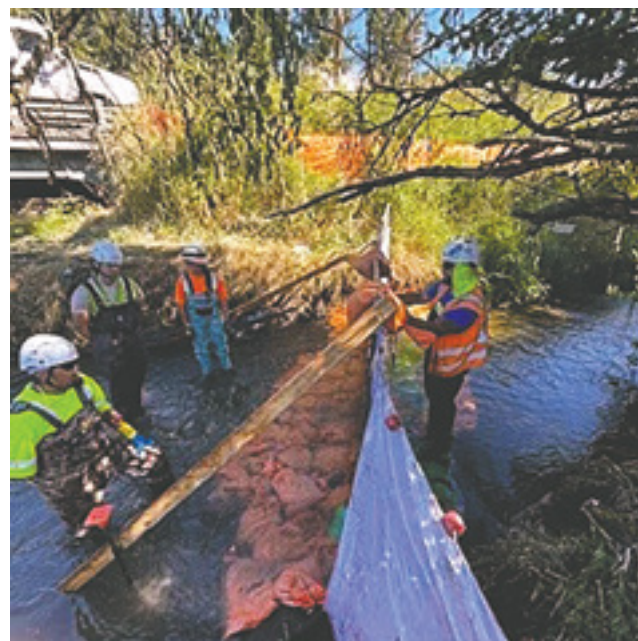
Crews install fine mesh nets to help exclude or capture fish in Hylebos Creek during the 2023 fish window.
